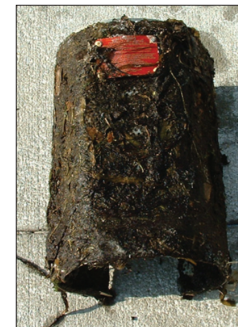
Intake screen clogged with aquatic weeds.
